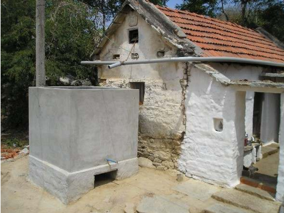
Domestic rooftop rainwater harvesting structure for a village house
