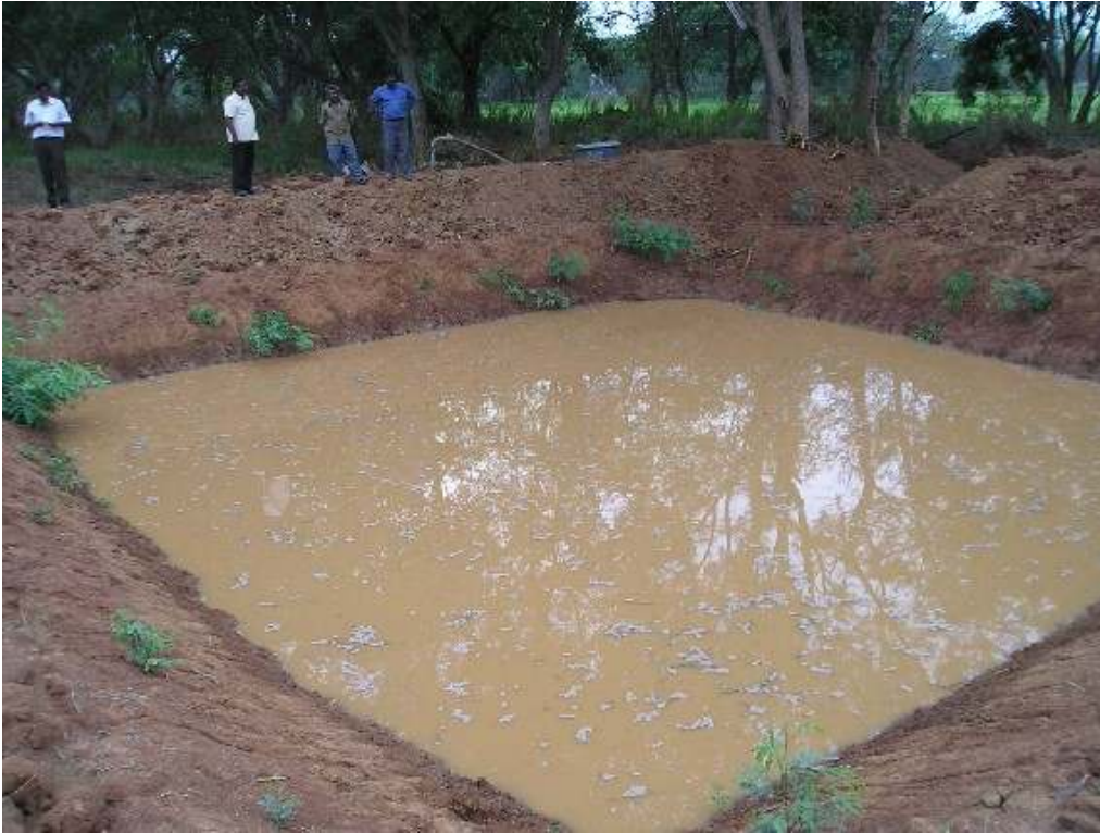
A farm pond next to a bore well, dug for recharge purpose
