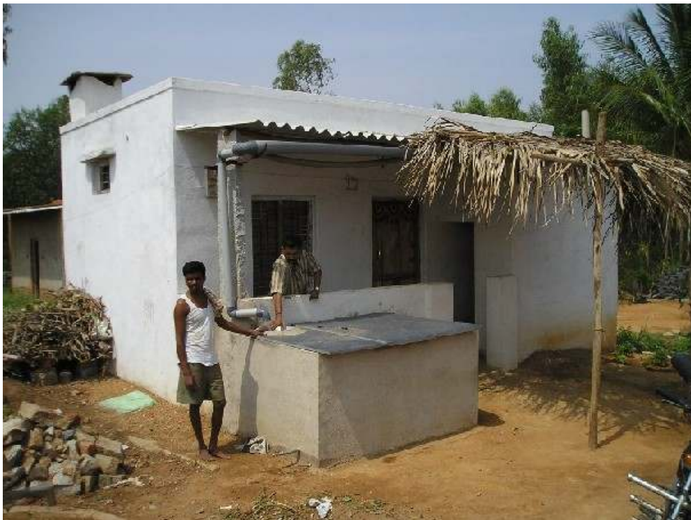
Rooftop rainwater harvesting system for a village house
